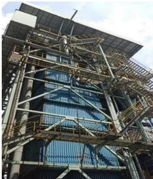
Gambar 1. Boiler Tipe Circulation Fluidized Bed (sumber: PT. Bukit Energi Servis Terpadu)
