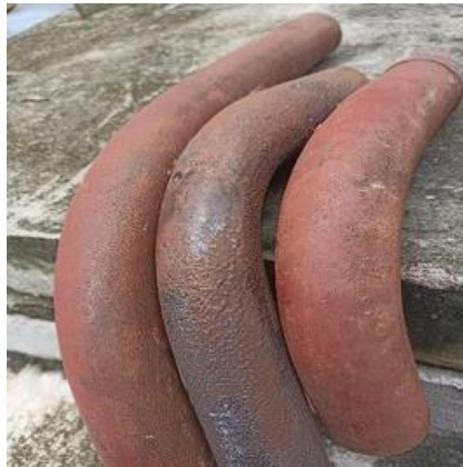
Gambar 2. Sampel pipa elbow superheater 90°
