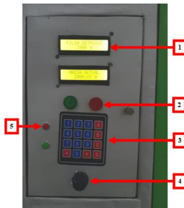
Gambar 7. Box panel kontrol
